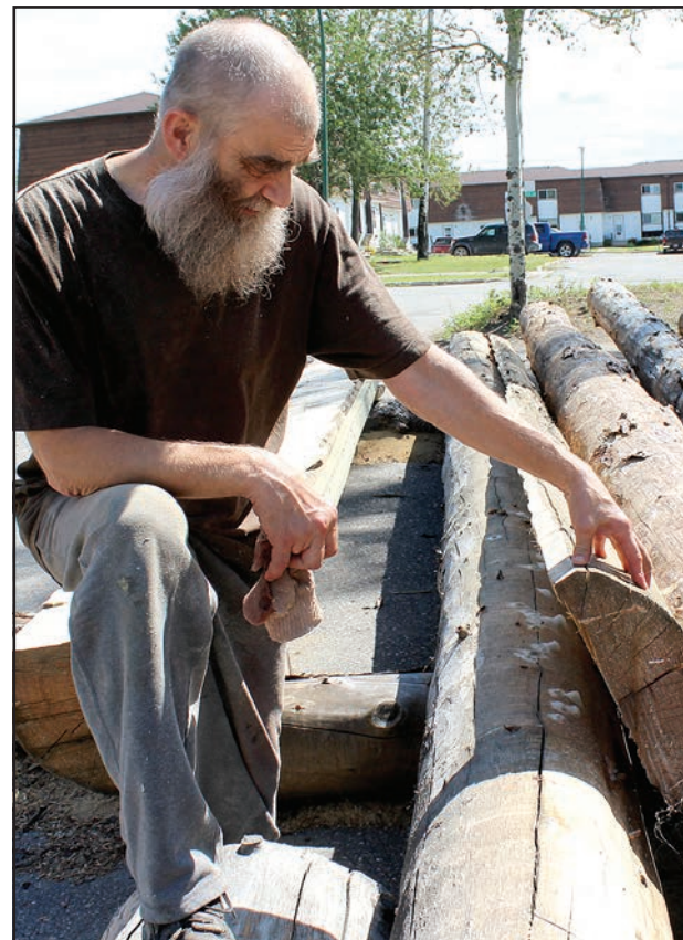
Friesen shows what slabs will look like for the log replacement project at the Heritage North Museum.
